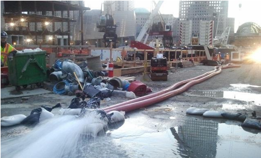
Photo: TITAN and Marine Pollution Control mobilized high-capacity pumping systems at the site of the World Trade Center memorial and museum in NYC.
