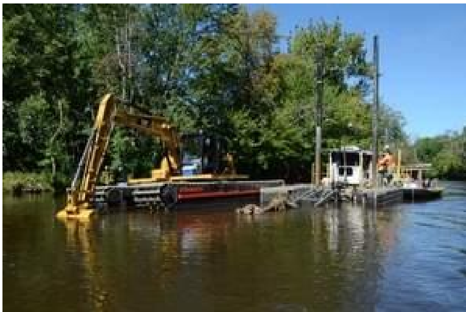
Photo: Site of a dredging operation in the Kalamazoo River between Historic Bridge Park and Battle Creek on Thursday. / John Grap/The Enquirer
