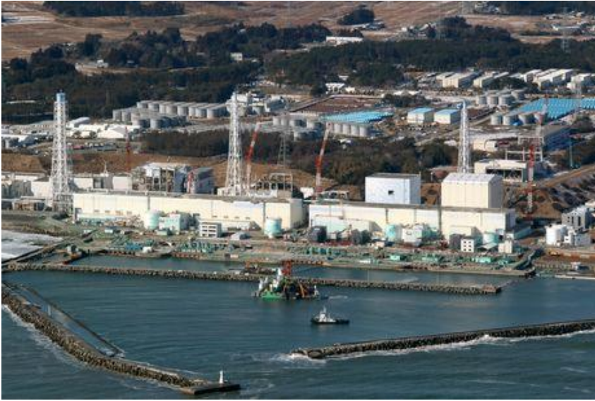
Photo: Workers begin pouring cement onto the seabed at the Fukushima No. 1 nuclear power plant on Feb. 28. (Eiji Hori)
