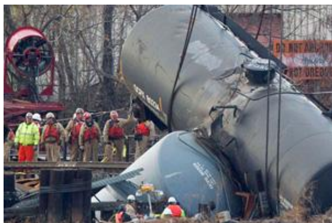
Photo: Work crews prepared to hoist the derailed tanker cars from the Mantua Creek in Paulsboro.
