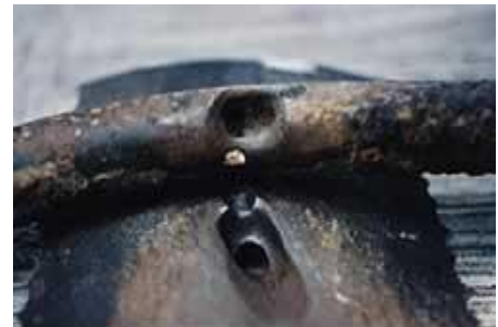
Corrosion and hole in larger gas pipe caused by smaller water pipe on top. Photo courtesy of Jose M. Malo, Electrical Research Institute, Mexico. Source: http://www.corrosion-doctors.org/Localized/sewer.htm ; accessed May 5, 2006.
