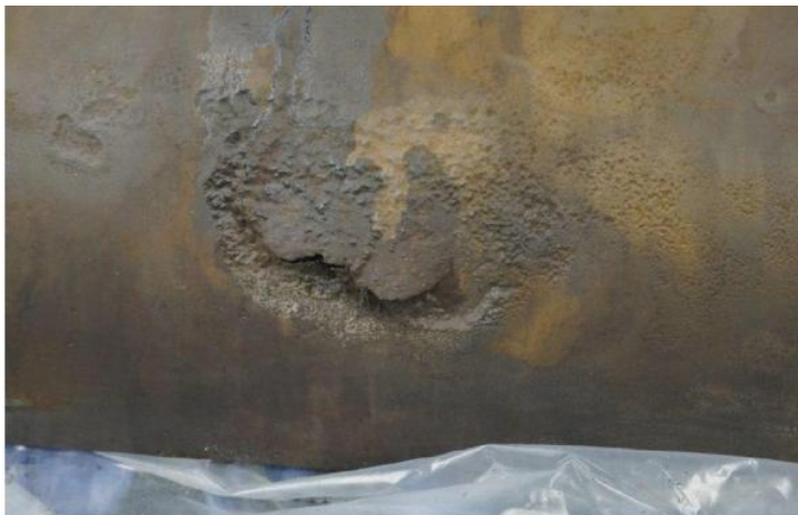
Pipe External Surface at the Line 901 Failure Site
