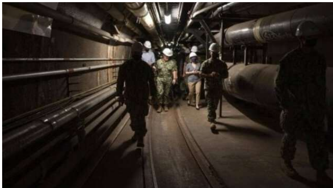
Photo: A tour of the lower access tunnel at Red Hill. The white large-diameter PVC line at top center-left is the AFFF retention line (USN)
