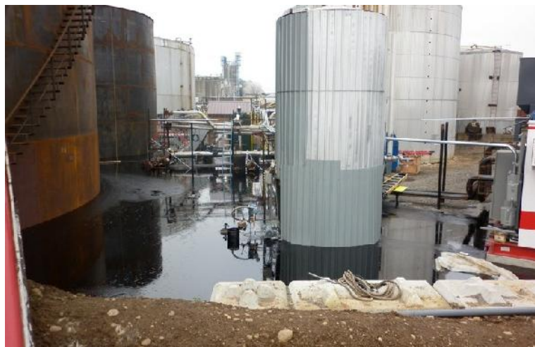
Photo: A tank failed at Albina Asphalt, spilling 220,000 gallons of asphalt oil into a containment area. (The Southwest Washington Clean Air Agency)
