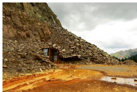
Photo: The opening to the Kohler Mine that has been bulkheaded August 13, 2015 along the Red Mountain Pass. Although bulkheaded, the mine is still slowly leaking water that is making its way into the Animas River.
